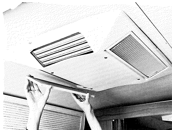
Air Conditioner Ducts and Filter
