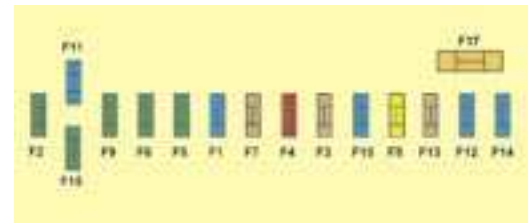
Fuses in the glovebox
